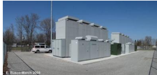
Sodium Sulfur Battery 2 MW
