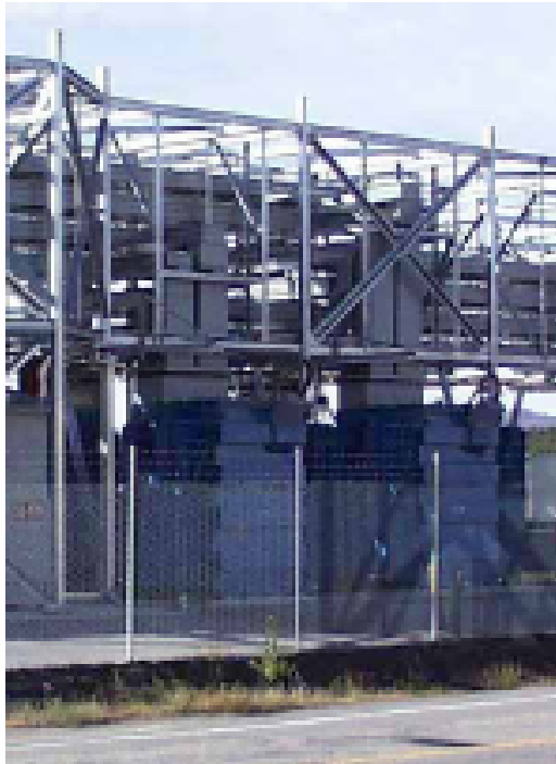
Typical H.V. Transformer
